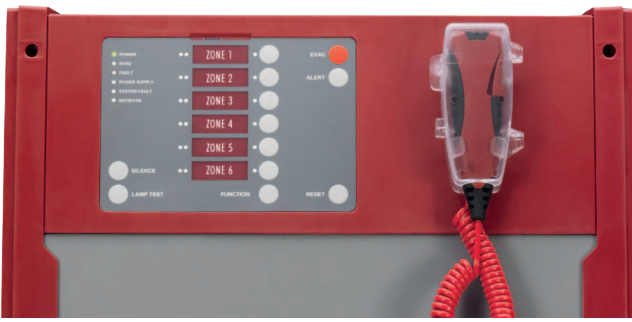
Control/Indications & Firemen microphone at access level 2
